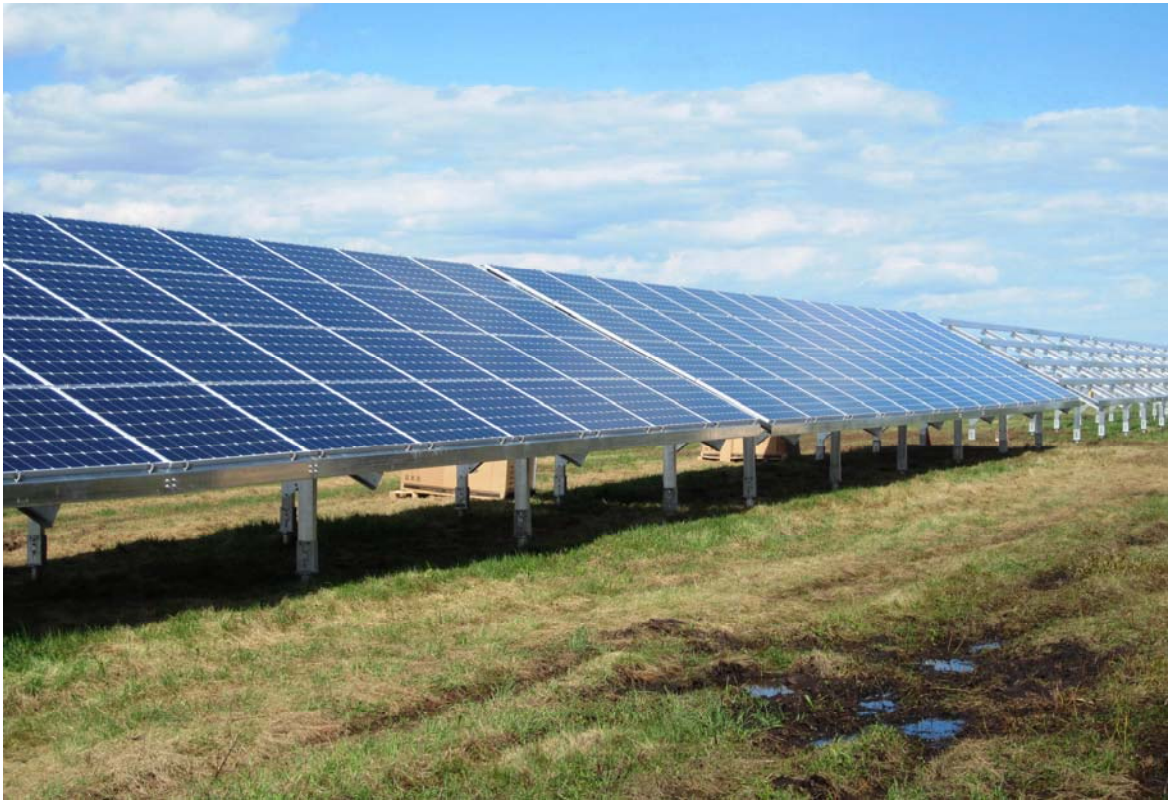
Figure 3.2 Photograph of Typical Solar PV Module Installation
